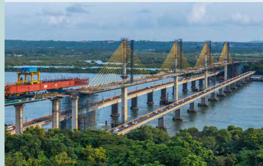
Project: Mandovi Bridge, India Stay Cable: Dywidag-Systems International GmbH (DSI), Germany Photo: DSI-Bridgecon
