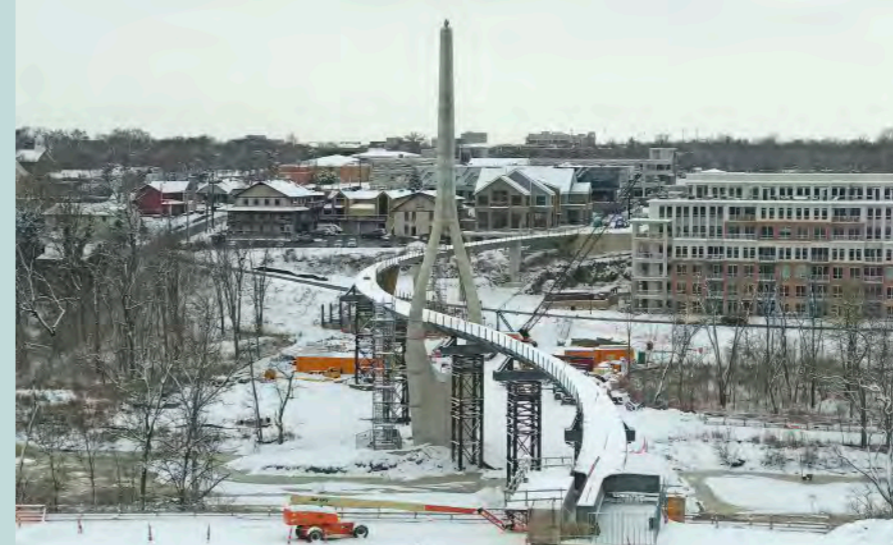
Project: Dublin-Ohio-Bridge, City of Dublin, Ohio, USA Stay Cable: Redaelli, Italy; Photo: Crawford Hoying
