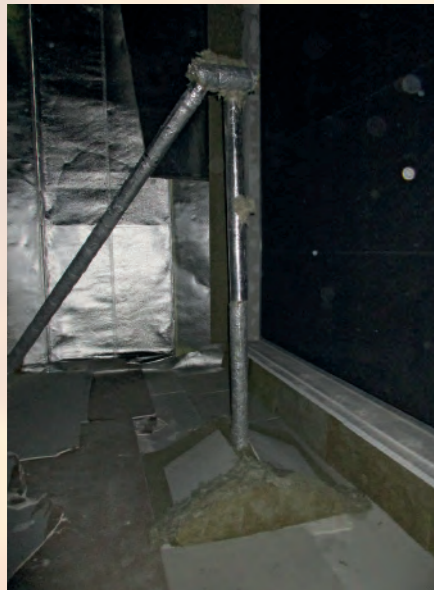
Radiation measurement on an 'E90' curtain
