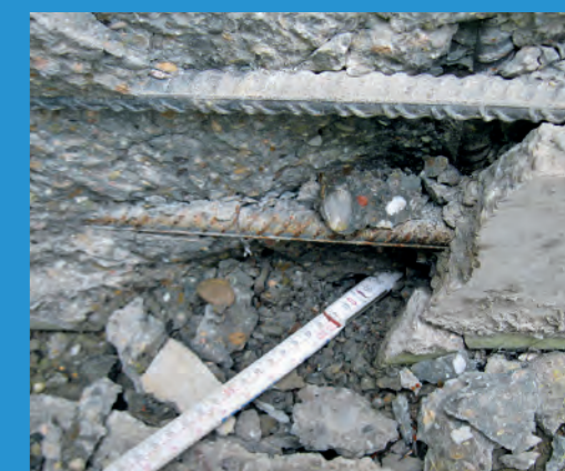
Uncovered concrete reinforcement steel
