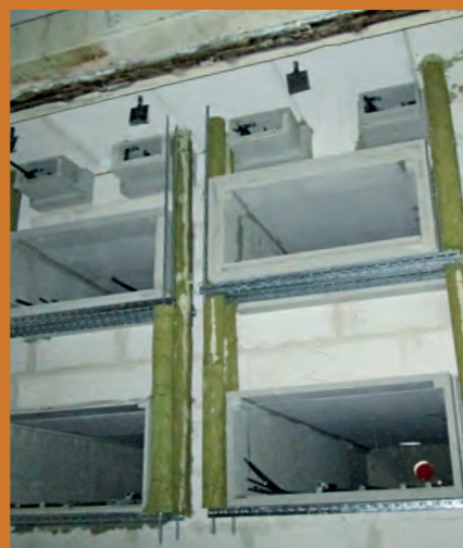
Installed service ducts
